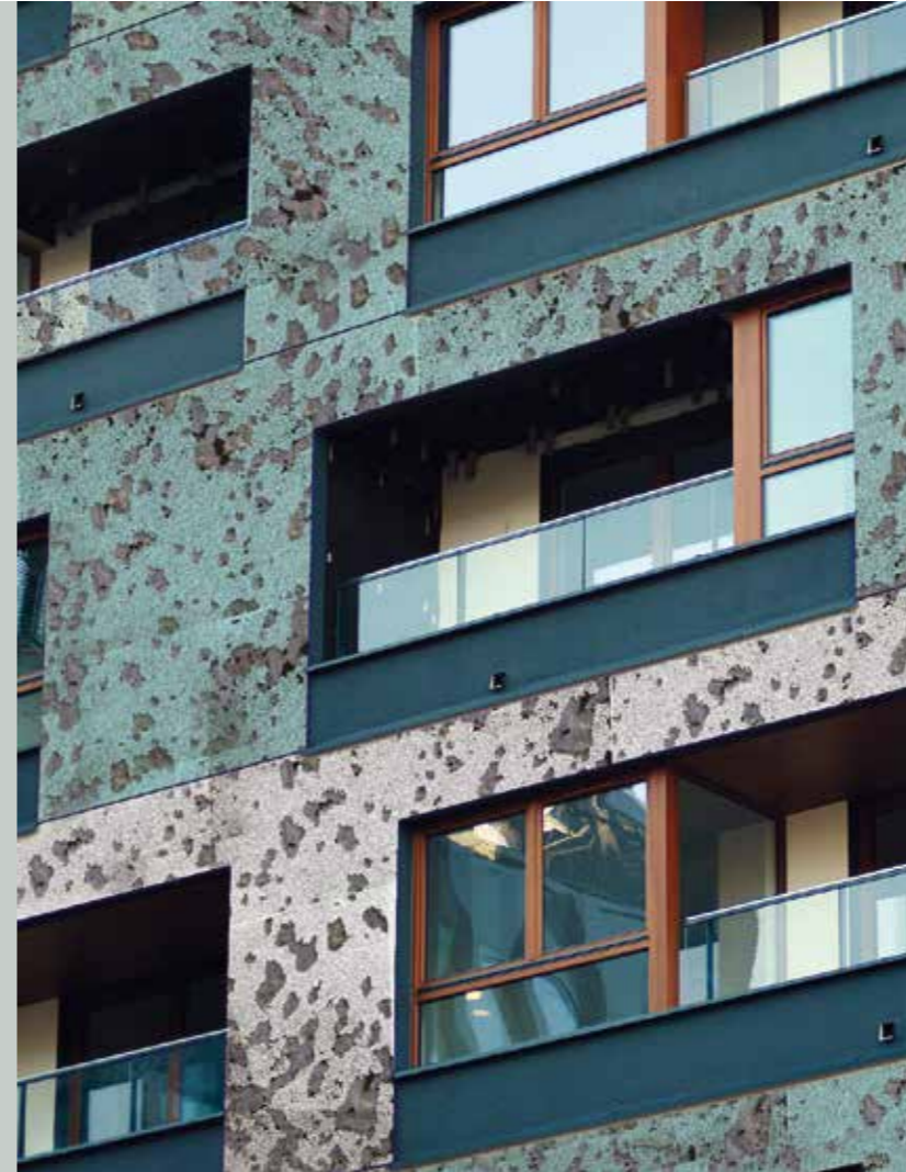
Hailstorm on External Thermal Insulation System
